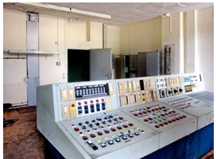
The plant control room. Photo Günther Schäfer - Alexis Forum
